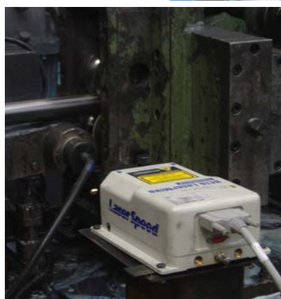
Cutting Control— Tube Mill
